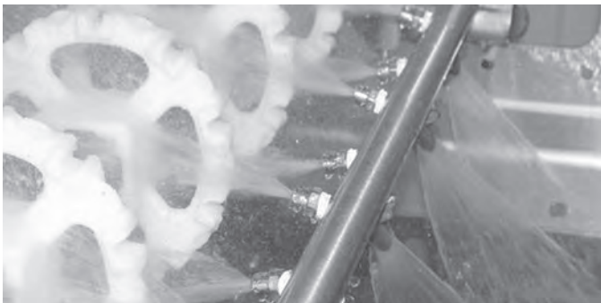
Figure 164: Spray pattern designed to clean of belt underside, sprockets, and shaft
