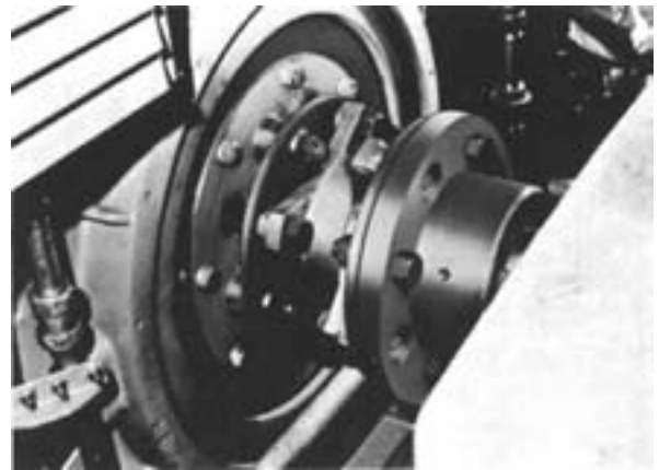
CMR coupling between engine and reciprocating compressor.
